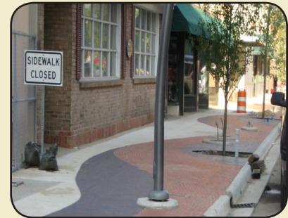
The sidewalk is taking shape along Michigan Avenue. The bricks are intended to mimic the movement of the river, as selected by Battle Creek citizens during the public input process.
